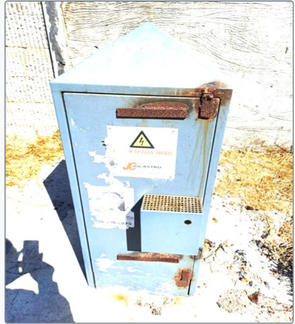
Multiple Entry Points: Vandals have compromised both doors despite welding.
