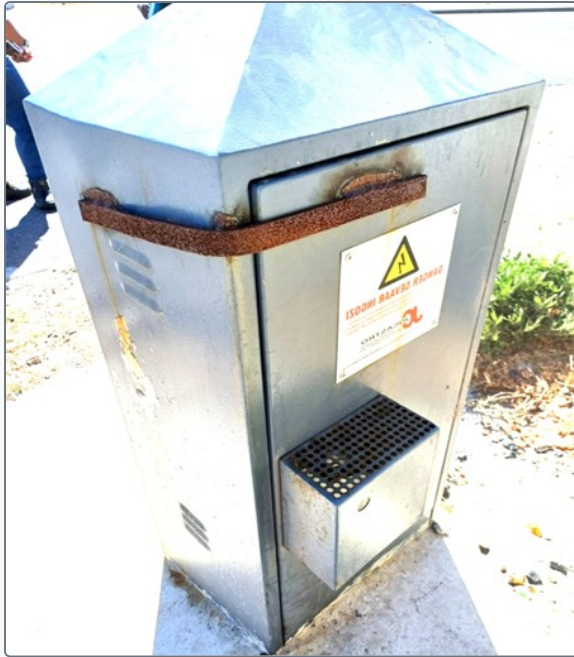
Welded & Broken: Kiosk door welded shut by authorities, then broken open by vandals.
